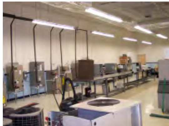
Heating and Air Conditioning Classroom
